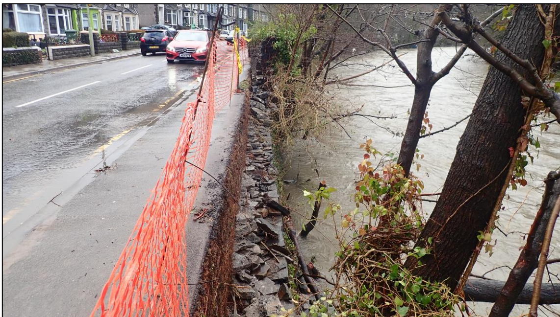
Figure 5: Collapsed river wall (NFD) on Berw Road following Storm Dennis (captured by RCT's Flood Risk Management team on 17 th February 2020)
